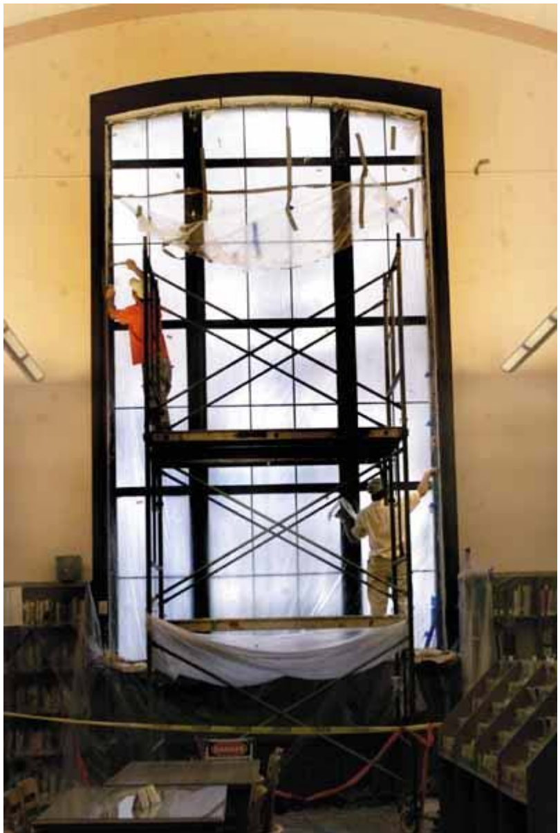
Workers replace insulation around one of the larger windows at the DeKalb Public Library on Thursday morning. Chronicle photo HOLLY LUNDH
