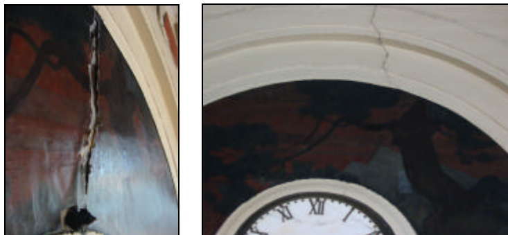
Above Left: Detail of the structural crack in the semi-circular doorway mural before treatment.. Right: The crack after treatment.
